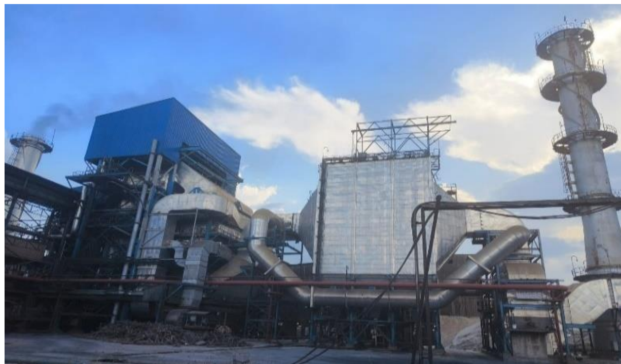
Figure 1. Water tube isgec yipe boiler
